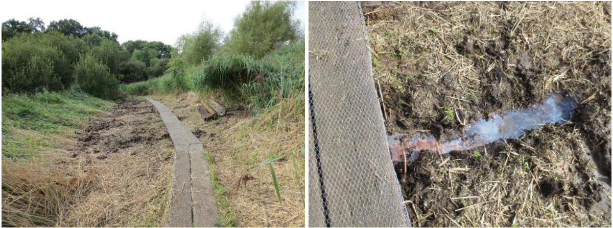
September 2012. Problems of waterlogging of boardwalk in fen needing remedial drainage work
