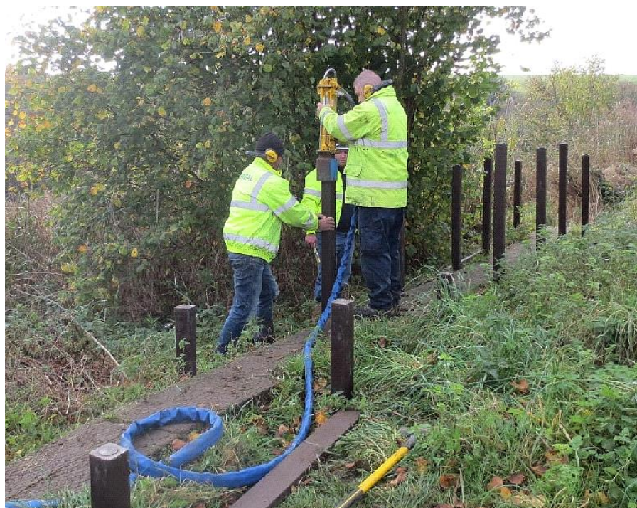
Recycled plastic boardwalk construction in progress at start of path through fen, 05.11.2014.
